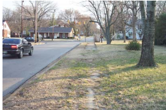
Sidewalk in Poor Condition
